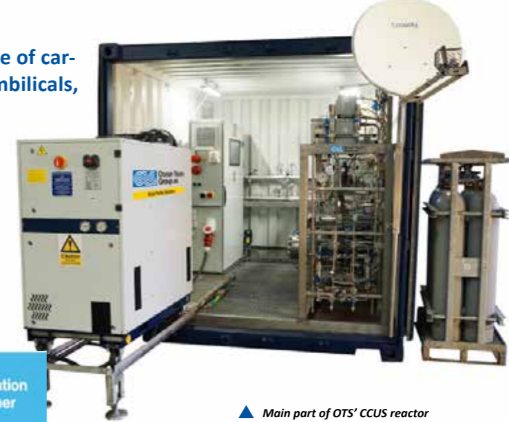
▲ Main part of OTS' CCUS reactor
