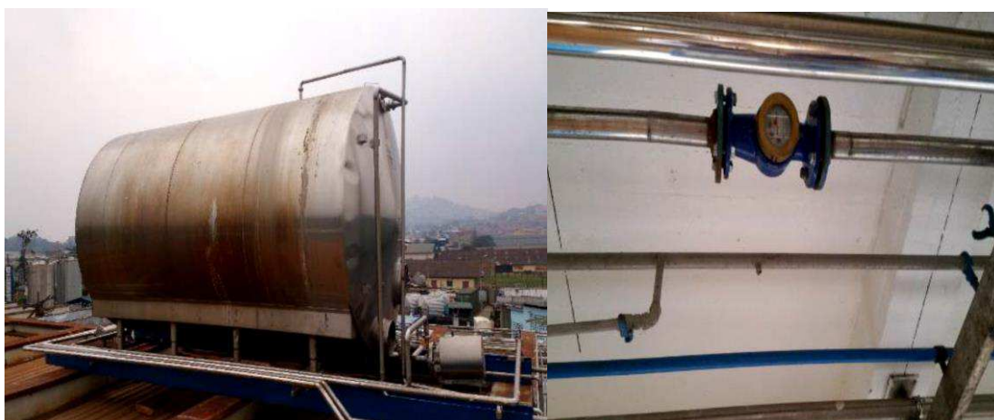
A recovery tank installed to recover cooling water and a meter installed to measure recovered water
