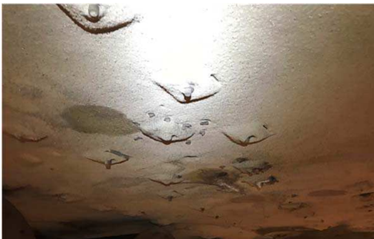
Figure 6.3-4 Area where fire protection has deteriorated.
