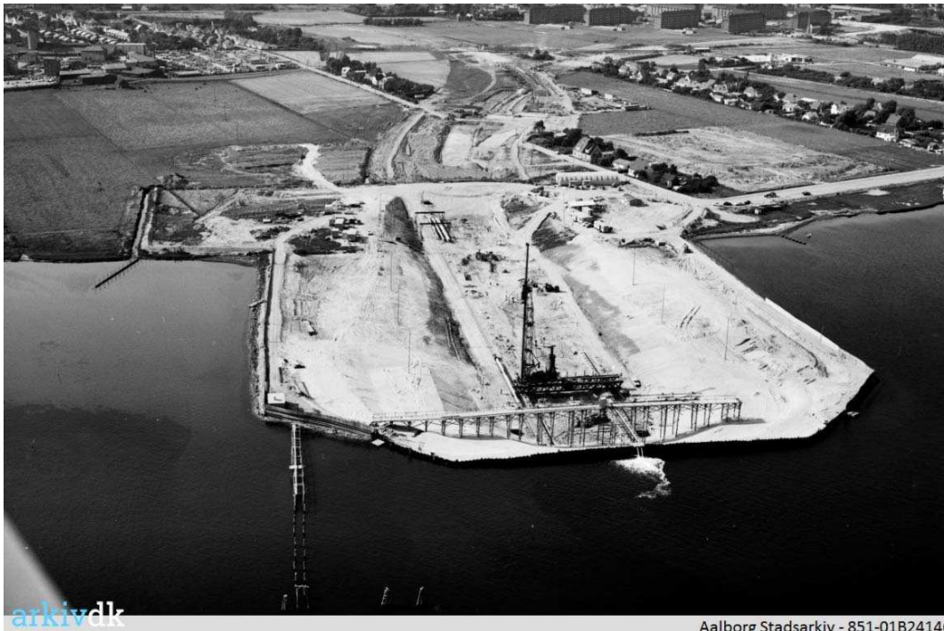
Figure 4.3-1 Dry pit at northern shore for casting of in-situ tunnel, portal building and ramp.
