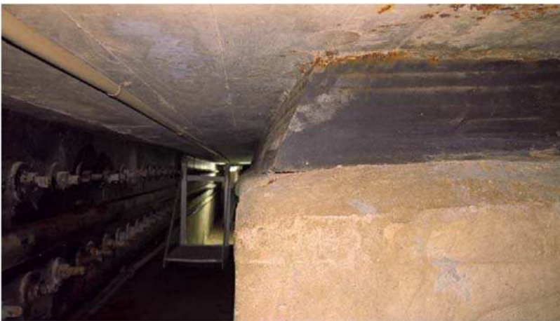
Figure 4.1-3 Elastomeric bearing at the northern portal building.
