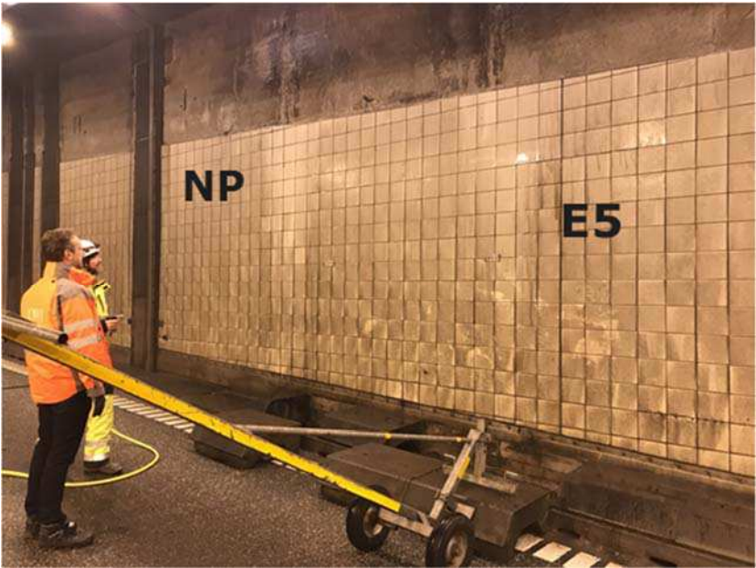
Figure 6.7-1 Closure joint between Northern Portal (NP) and Element V (E5) before removing tiles and concrete in order to inspect the reinforcement.
