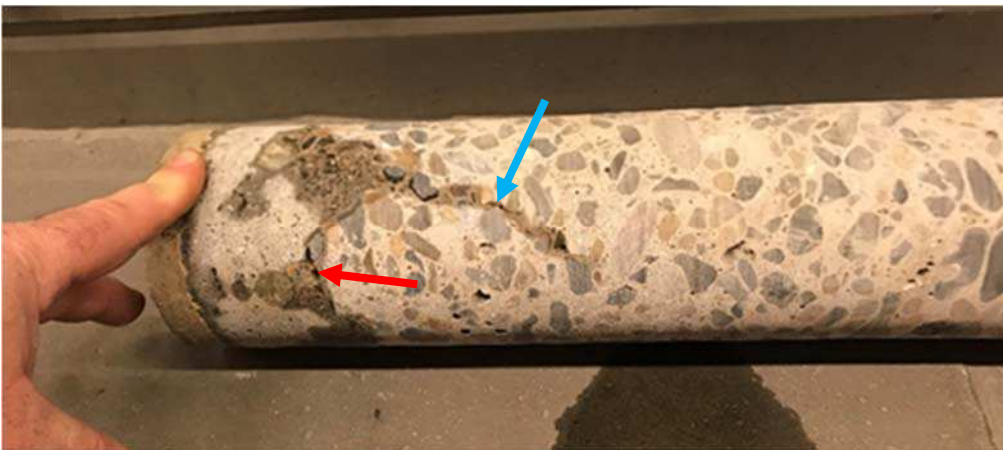
Figure 6.3-2 Core extracted from roof. The concrete is cracked both at the interface between repair and original concrete (red arrow) as well as within the original concrete (blue arrow).
