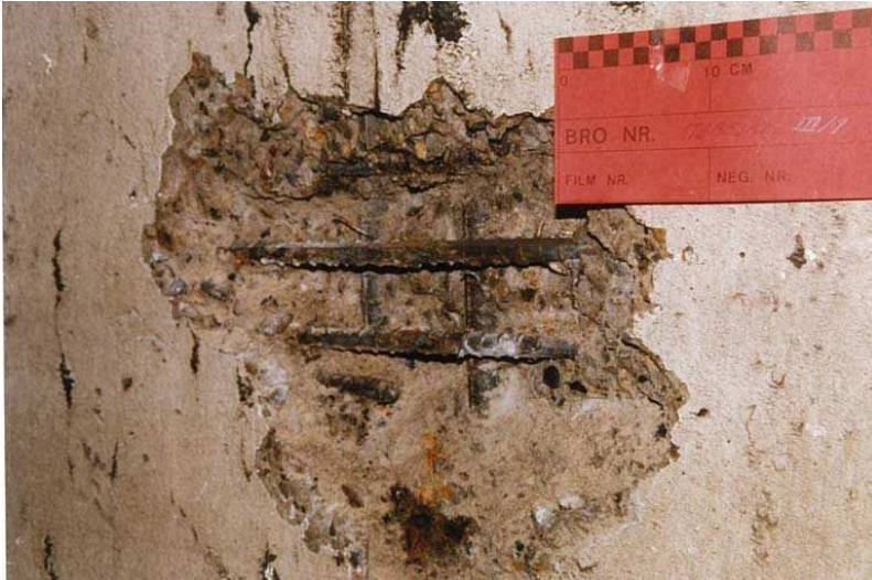
Figure 4.5-1 Reinforcement corrosion from inspection in 1988.
