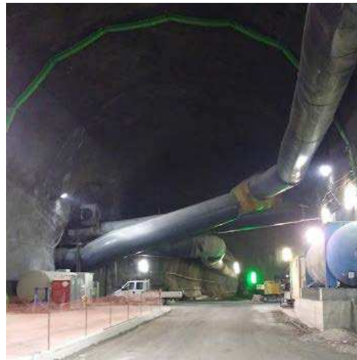
The cavern where the machinery is assembled
