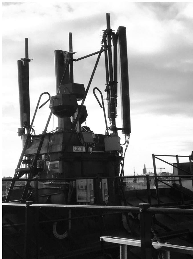
Figure 4. Group of base stations located 6 m from balcony outside tower. Photo taken from the balcony.
