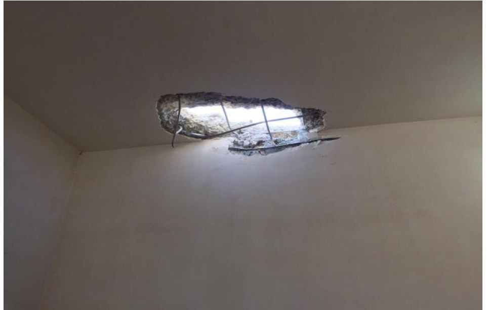
Picture of hole on the ceiling of a house due to mortar attack.
