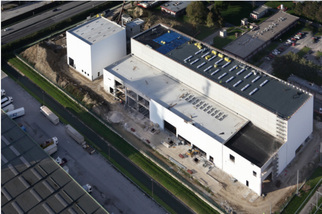
PRIMA building for the Neutral Beam Test Facility under construction at Padova in Italy
