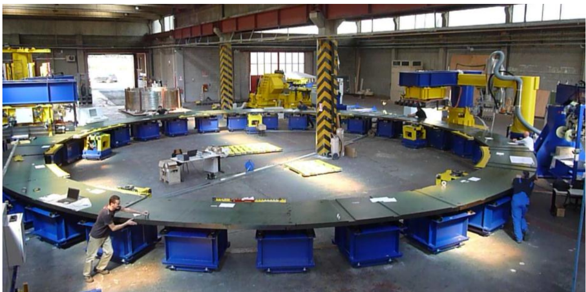
Tooling for the Poloidal Field (PF) coils under assembly for acceptance testing. The coils will have to be manufactured on the ITER site since they cannot be transported due to their size
