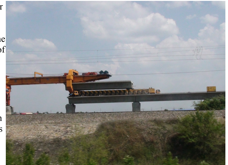
Picture 7: Image source - Wikimedia commons. Image depicts the construction of elevated conventional rail. This method can be used for magnetic track.
