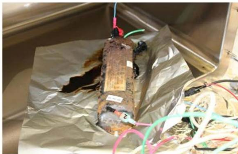
Figure E.7. The light ballast that burst during the emission test with electrical load
