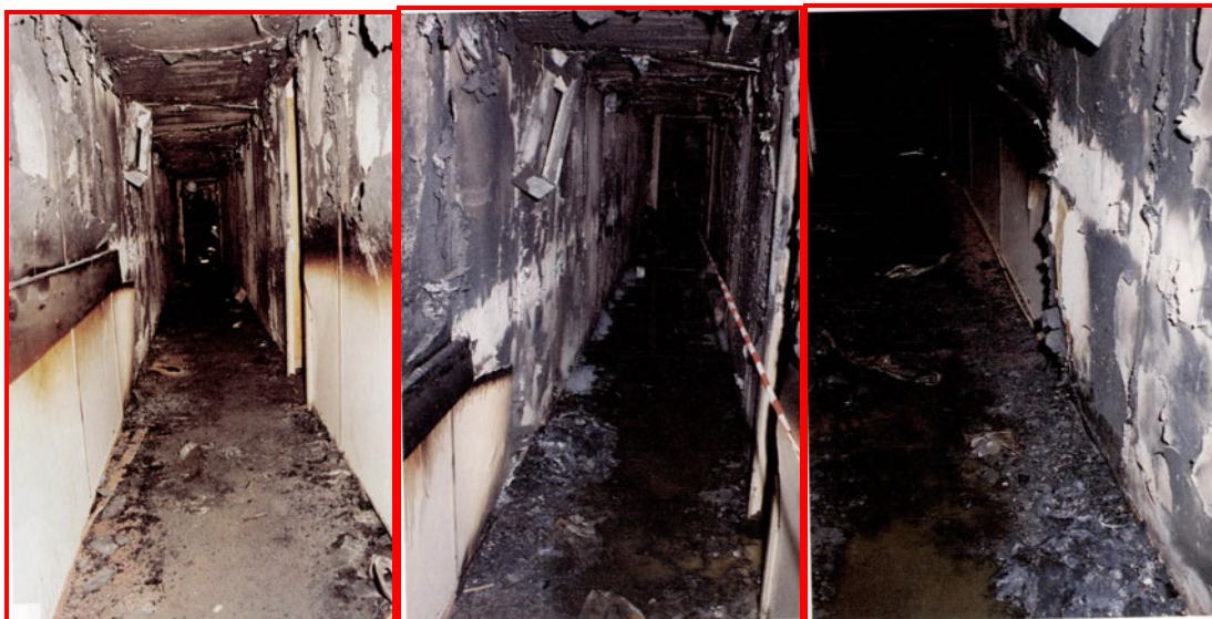
Figure 10. Three photographs showing damages in the hallway on deck 3, on starboard side of the ship, astern of staircase D s (2 SB). The door opening, visible to the right in the picture on the left, leads in to cabin 219. Fire no. 2 (the main fire) was started in this hallway.
