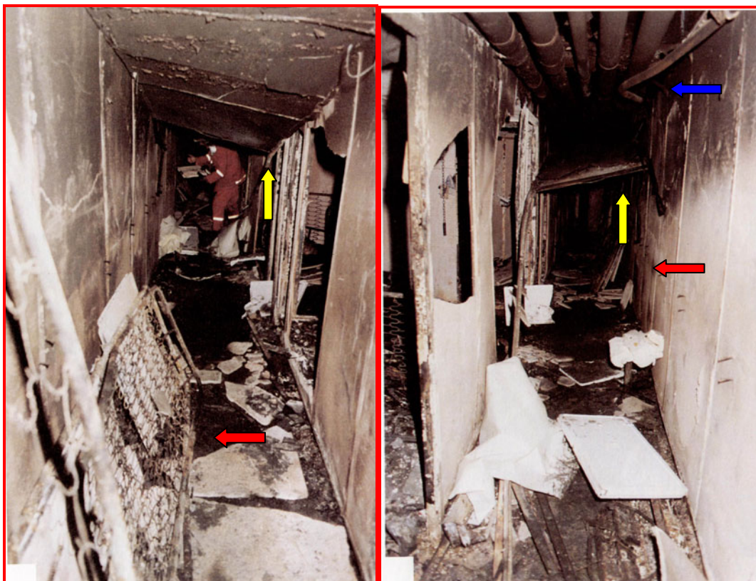
Figure 12. The two photographs show the location for the start of fire no. 3 (the hydraulic fire). On these photographs, the bed (indicated by a red arrow) that most likely has been used to ignite the hydraulic oil is visible. The blue arrow indicates the hydraulic pipe in question. The other pipes, set in the same ceiling section as the leaking hydraulic pipe, are unaffected by the fire. Note that only some parts of the ceiling section (indicated by a yellow arrow) that, prior to the fire, was covering the entire pipe zone has collapsed despite the fact that the entire corridor was involved in this fire which indicates that it was destroyed by hand before the fire.
