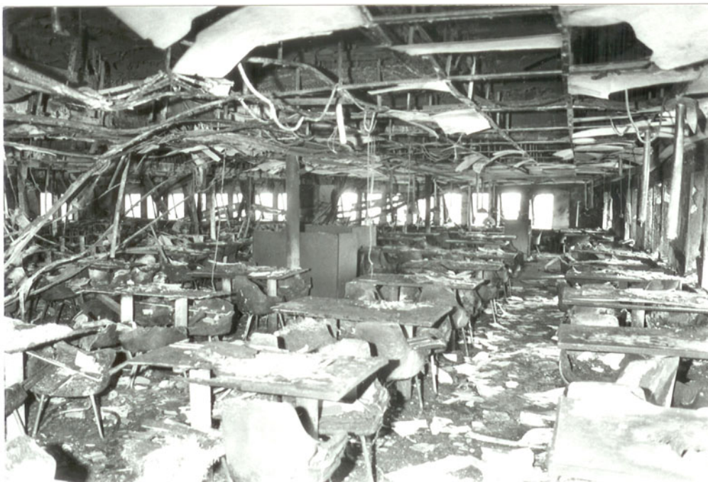
Figure 14. Photograph showing the restaurant in the front part of deck 6. The heavy fire damages are most likely the effects of fire no. 6.
