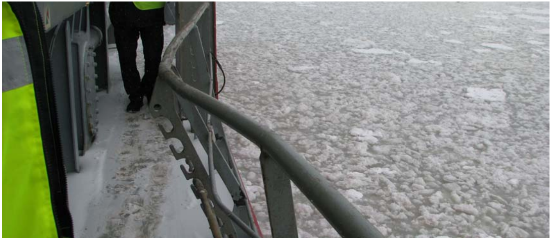
Figure 5. The railing damaged by the fallen container stack on the port side of the vessel.
