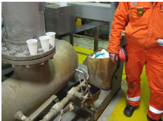
Figure A5.3 Sampling Point for Skjold
