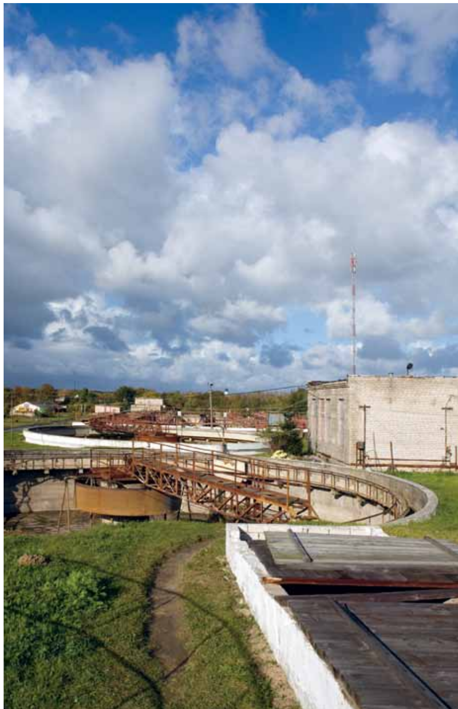
The technical systems at the 35-year old plant in Svetlogorsk are at the end of their service life.
