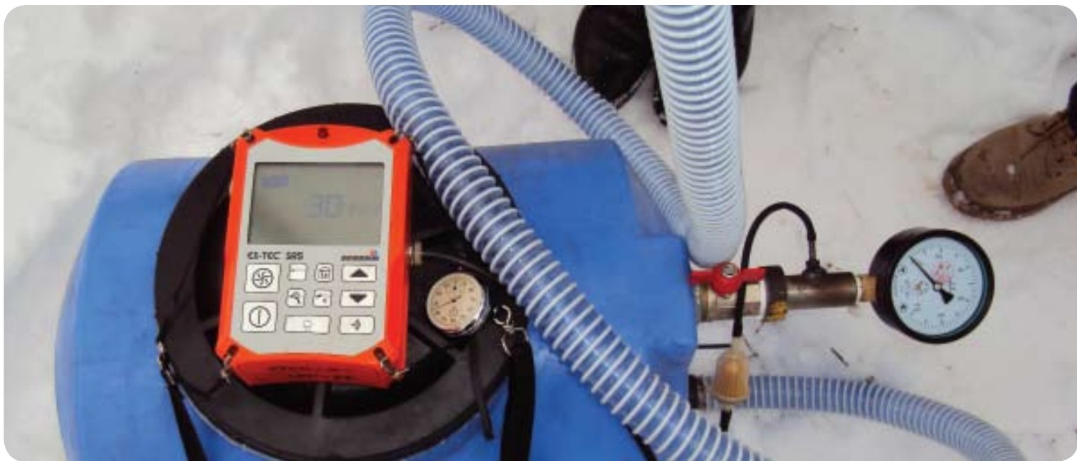
Measurement system for detection of gas leakage in the network.
