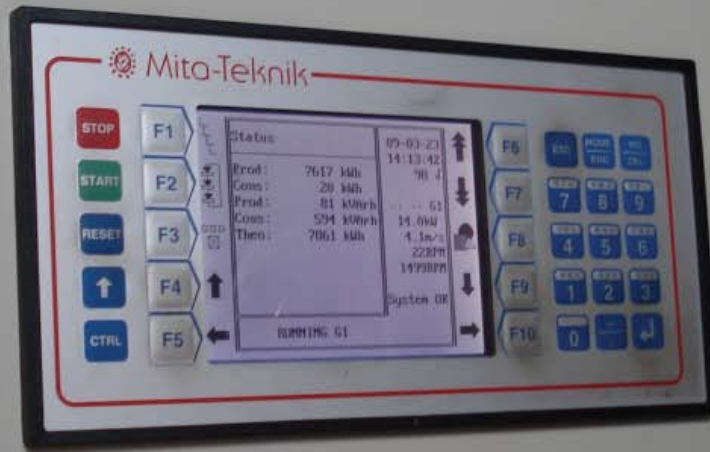
Presentation of the new installed equipment. The project is expected to be at full operation and capacity ultimo 2010.
