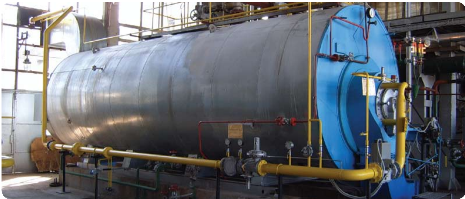
With the installation of new cogeneration technology the two plants will be able to reduce costs, increase competitiveness, and achieve more efficient fuel usage as well as a significant reduction of CO 2 emissions.
