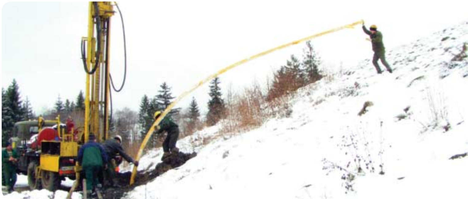
A system of pipes has been drilled into the landfills to collect and transport methane gas from the garbage heaps to gas generators.
