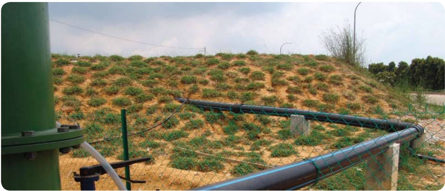
Gaspipes extracting gas from the landfill.
