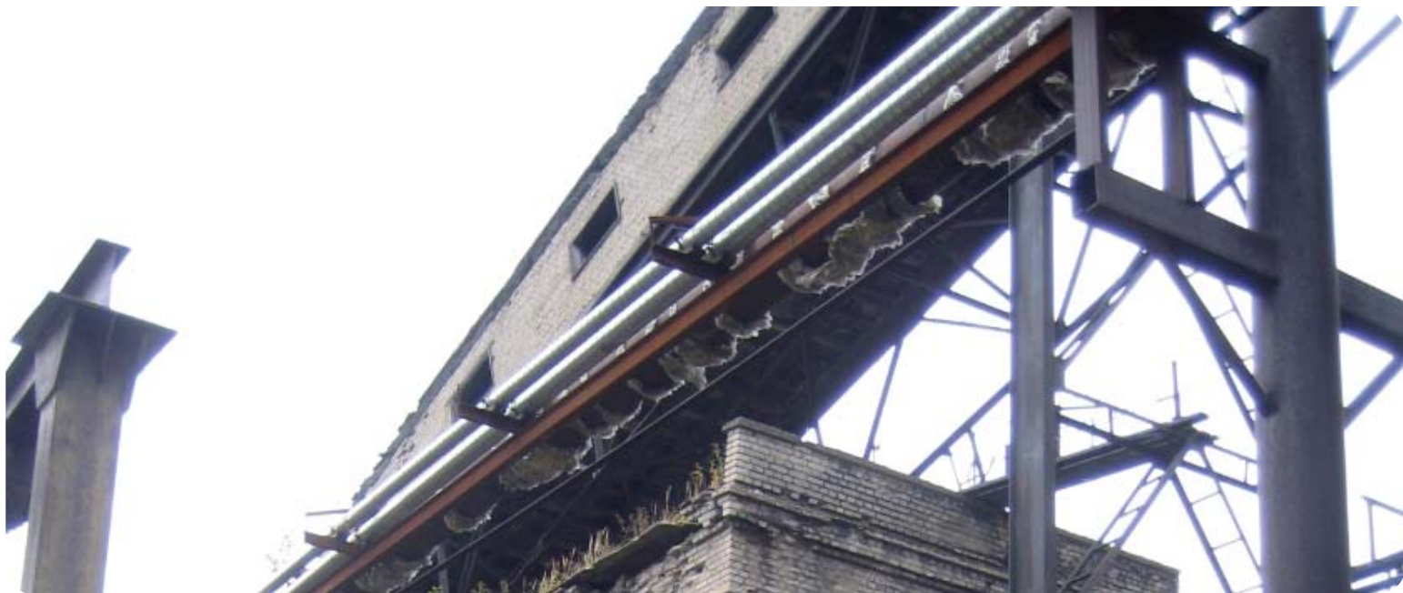
The biggest heating source in Priozersk is a mazut-fired combined heat and power plant established in 1936.
