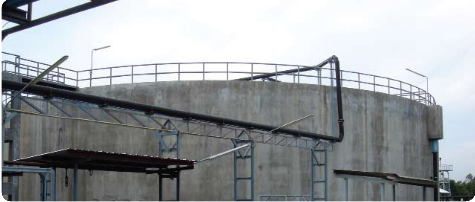
One of the tanks where bacteria digest the organic content in the wastewater and convert it to biogas.
