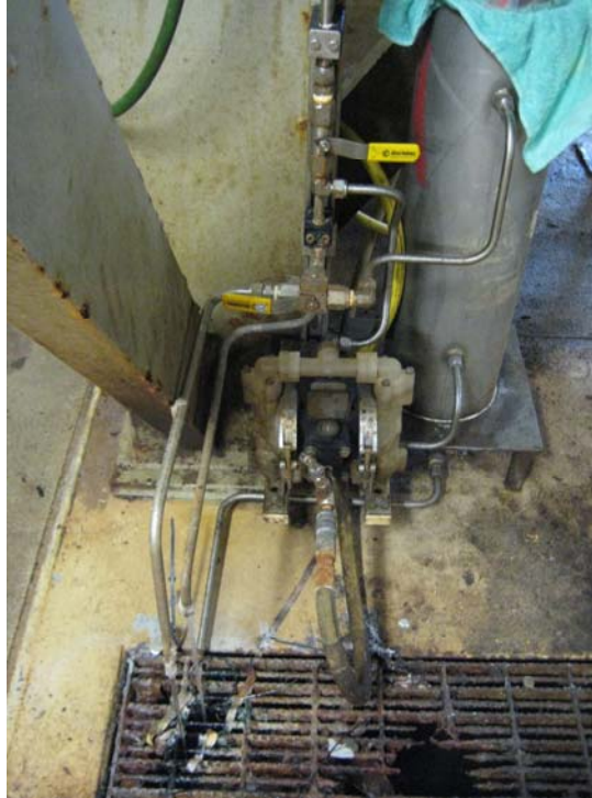
Figure A4.1 Sampling Point and Online Monitor Discharge, Dan FF
