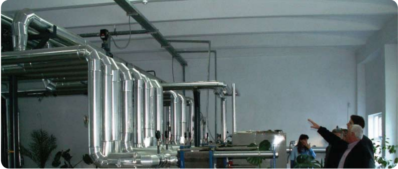
Presentation of heat exchangers in the substations.
