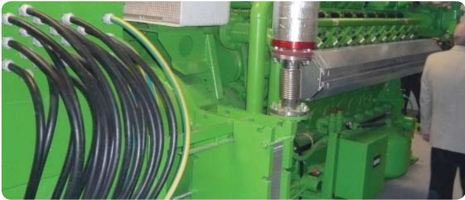
Poldanor biogas plant at the farm at Pawłówko. Manure and organic waste such as maize ensilage and slaughterhouse waste are mixed with slurry by which methane is produced and utilized.
