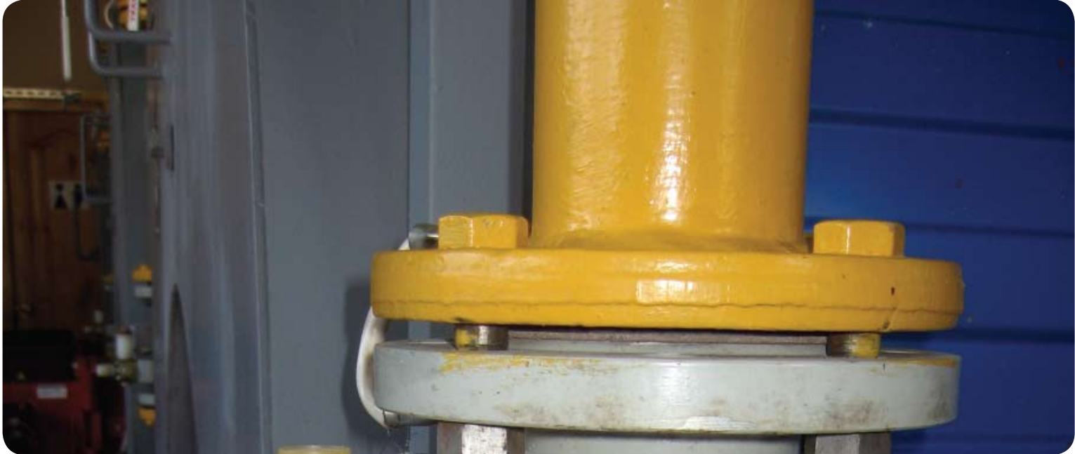
A new meter inside a boilerhouse measuring use of natural gas. An important task before calculating the GHG reduction.
