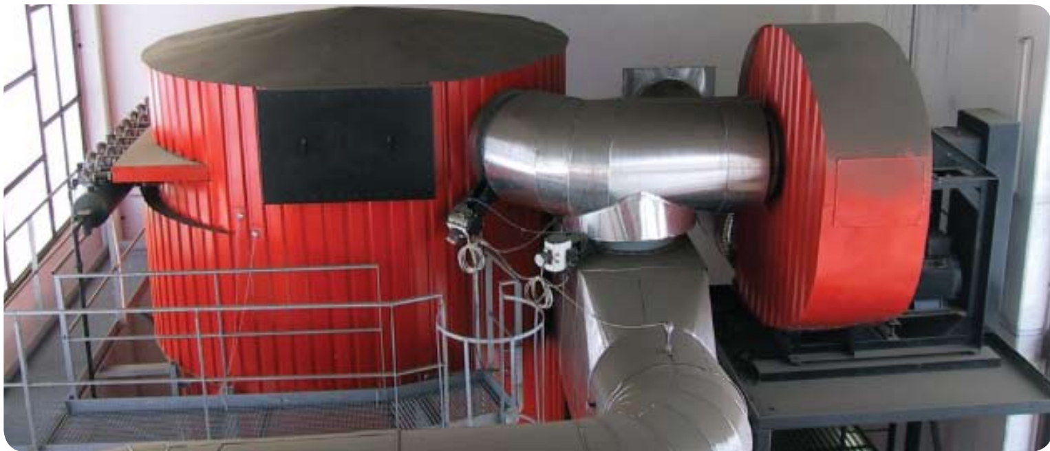
The applied technology replaces fossils fuels and combust natural residuals instead.
