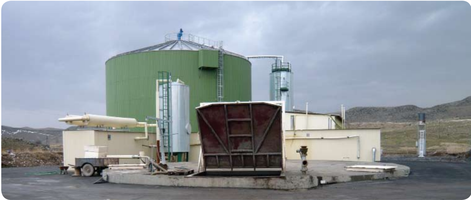
The embedded biogas technology is delivered by Denmark's Bigadan, and financed through the CDM mechanism.
