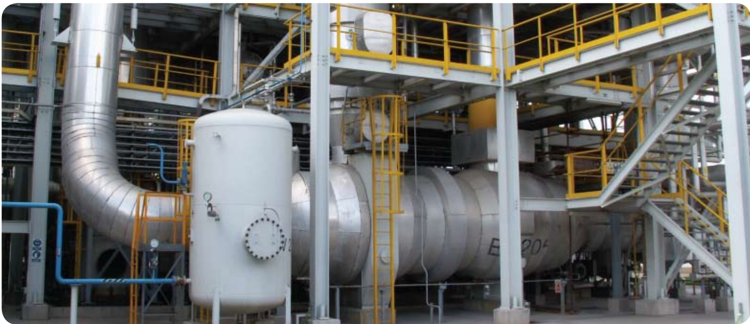
The project's aim is to reduce N 2 O emissions at the nitric acid plant of Lovochemie and provide additional environmental and social benefits.
