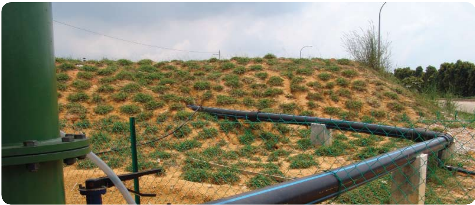
Gaspipes extracting gas from the landfill.
