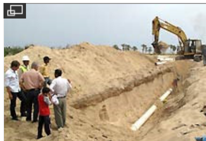
The ICRC is continuing to support construction work for the waste water treatment plant in Rafah.
