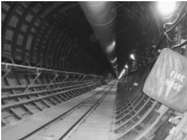
The nuclear “waste” storage facility at Yucca Mountain, Nevada. Though the subject of enormous hysteria, the products generated by nuclear fission include large amounts of precious metals. Japanese researchers consider such spent fuel to be one of the most valuable “ores” known today. The fusion torch technology will make it possible to deal with such radioactive materials.
