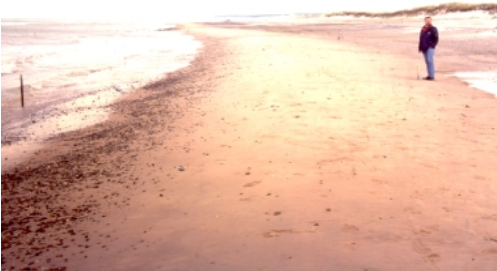
Figure 3: A "Jakobsen pipe" installed at Gammel Skagen on the Danish north sea Coast.
