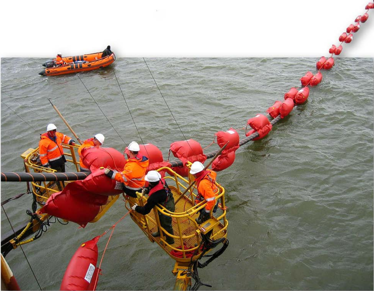
The laying of the NorNed cable between Norway and the Netherlands. Photo: Statnett
