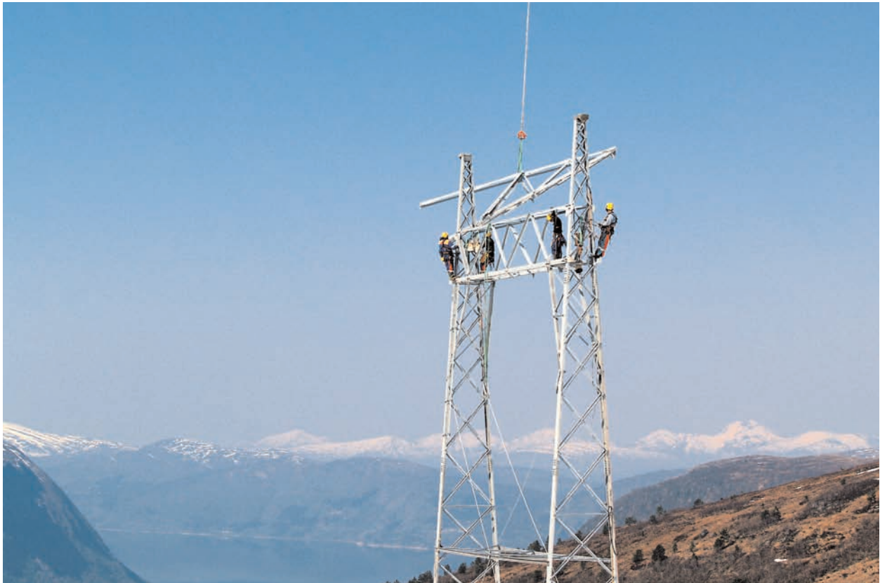
Construction work on a new 420 kV line at the Meisa mountain in Norway. Photo: Statnett
