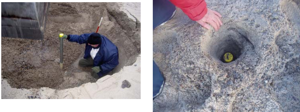
Figure 4.B: Left: The inventor of PEM Poul Jacobsen installs an additional tube in the beach (peaking). Right: The tubes are initially buried, so the top is around 30 cm below beach surface.
