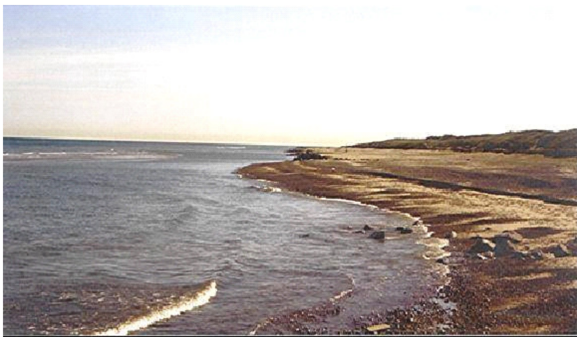
The PEM modules create a groin that catches long shore sand transport.
